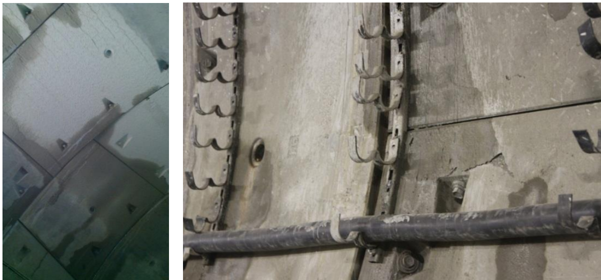
Figure 1. Infiltration through the reinforced concrete lining of the subway tunnel (photo taken by the authors)
