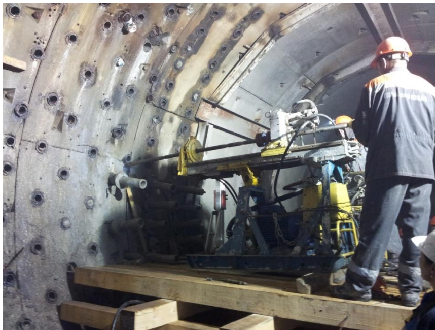
Fig. 4. Restoration of impermeability and load-bearing capacity of reinforced concrete linings through injection using immersed perforated injectors (photo taken by the authors)
