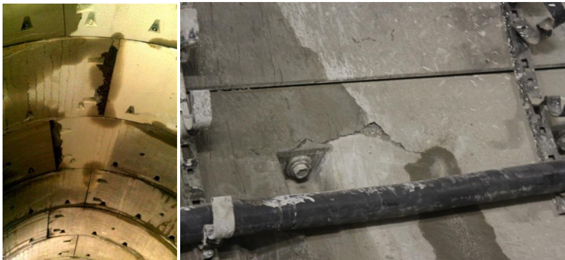
Figure 3. Cracks in the reinforced concrete blocks of the tunnel linings (photo taken by the authors)
