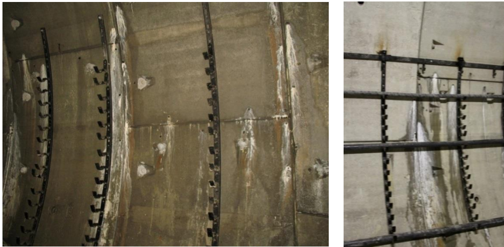
Figure 2. Efflorescence of calcite ( \text{CaCO}_3 ) – the product of leaching and carbonation of \text{Ca}(\text{OH})_2 from the concrete (photo taken by the authors)
