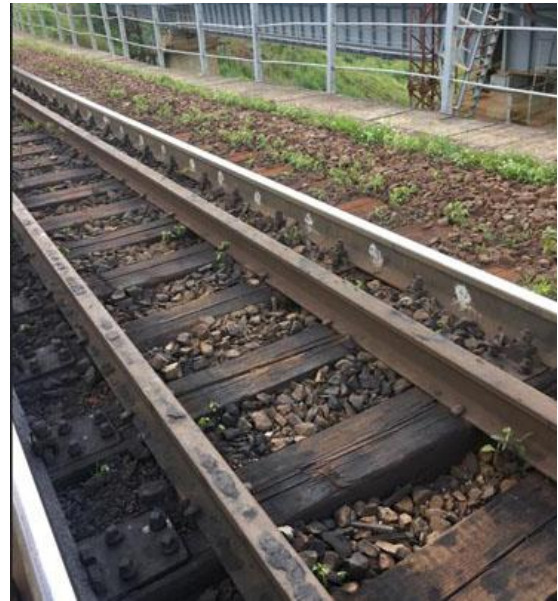
Figure 11. Defective sleepers (three or more in a row)
