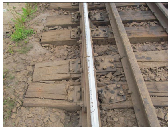
Figure 12. Defective rails on the bridge and its approaches
