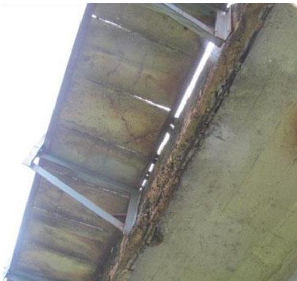
Figure 10. Defective reinforced concrete sidewalk blocks: leaching and deterioration of concrete, cracks, spalling
