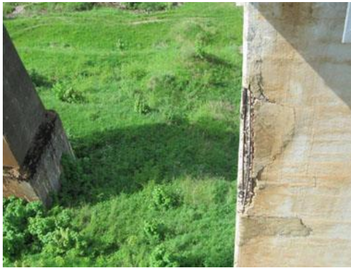
Figure 24. Freeze-thaw damage to concrete of reinforced concrete structures
