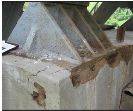
Figure 21. Loose bearing of the superstructure or bridge bearings
