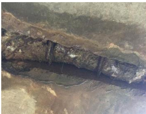
Figure 15. Freeze-thaw damage to concrete
