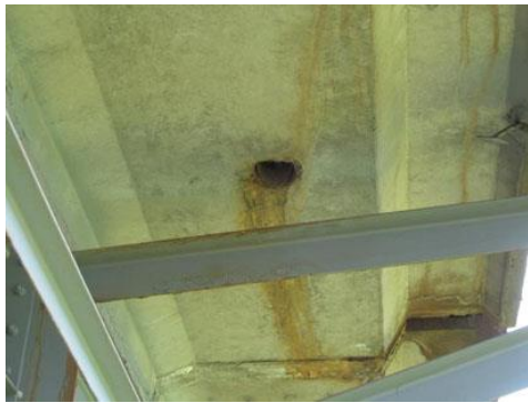
Figure 14. Defective or missing drainage pipes
