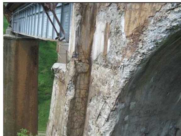
Figure 23. Freeze-thaw damage to the concrete of reinforced concrete abutments
