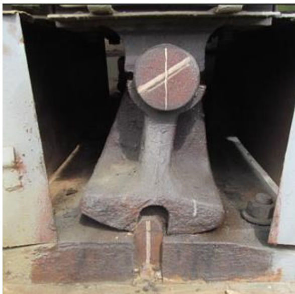
Figure 20. Deviation from the design relative position of the rocker and the base plate
