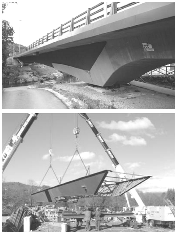
Fig. 19. Bridge over the Sella River in Cangas de Onis, Spain – general view and construction stage [10]
